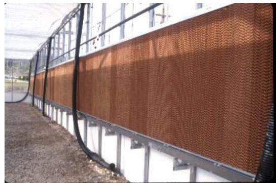
Picture 2 - Evaporative Cooling Wall
